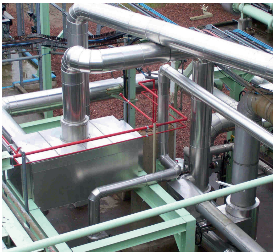
Operating as a reboiler in the solvent recovery column at Dow Wolff Cellulosics, Compabloc offers a substantial increase in capacity compared with the shell-and-tube heat exchanger it replaced.
