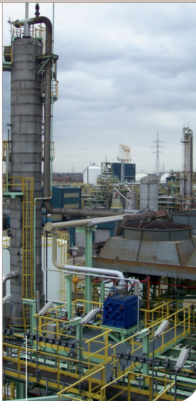
Installed as a condenser in a solvent recovery column at Dow Wolff Cellulosics, the Compabloc compact heat exchanger is visible next to the air coolers.
